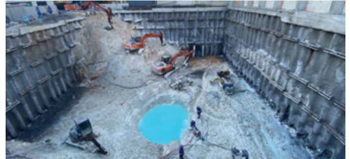
The basement shows white kaolin clay to final level, with restricted excavation techniques.
